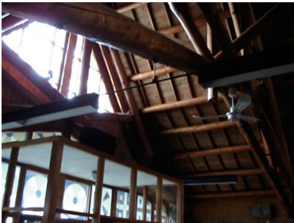
Figure 16. Interior of Saint Michael's Church. See details of woodcraft of untreated and exposed beams.
